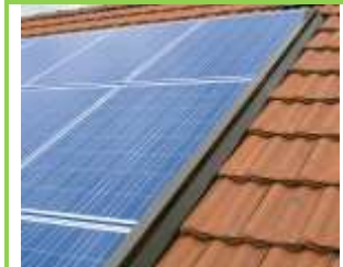
Polycrystalline PV array
